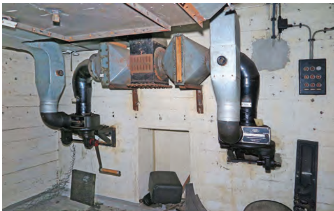
Ventilation equipment within Eidelstedter Weg. The emergency hand-cranking handle can be seen on the left-hand side
